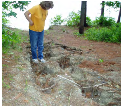
Soil erosion like this brings excess phosphorus into lakes.
