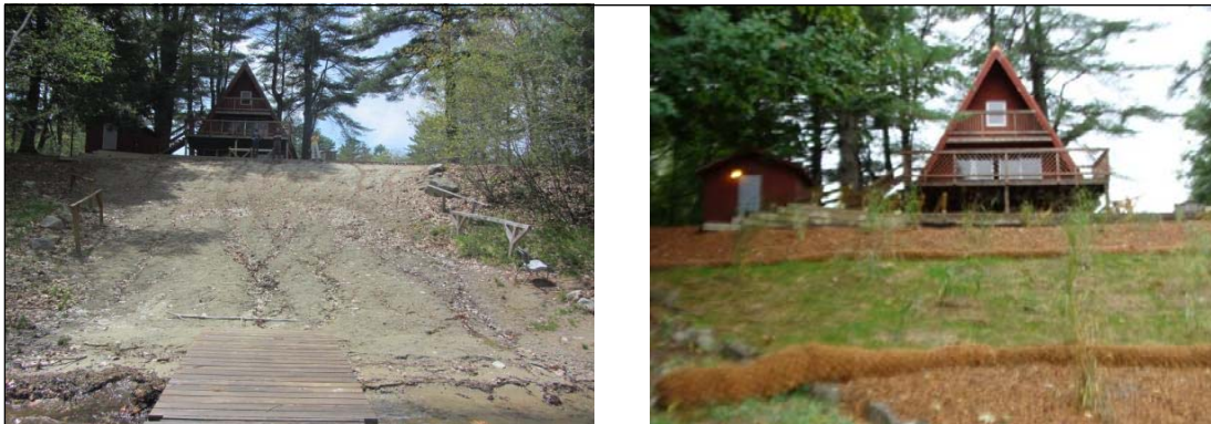
Remediation of the highly eroding "ski beach" at a youth camp
