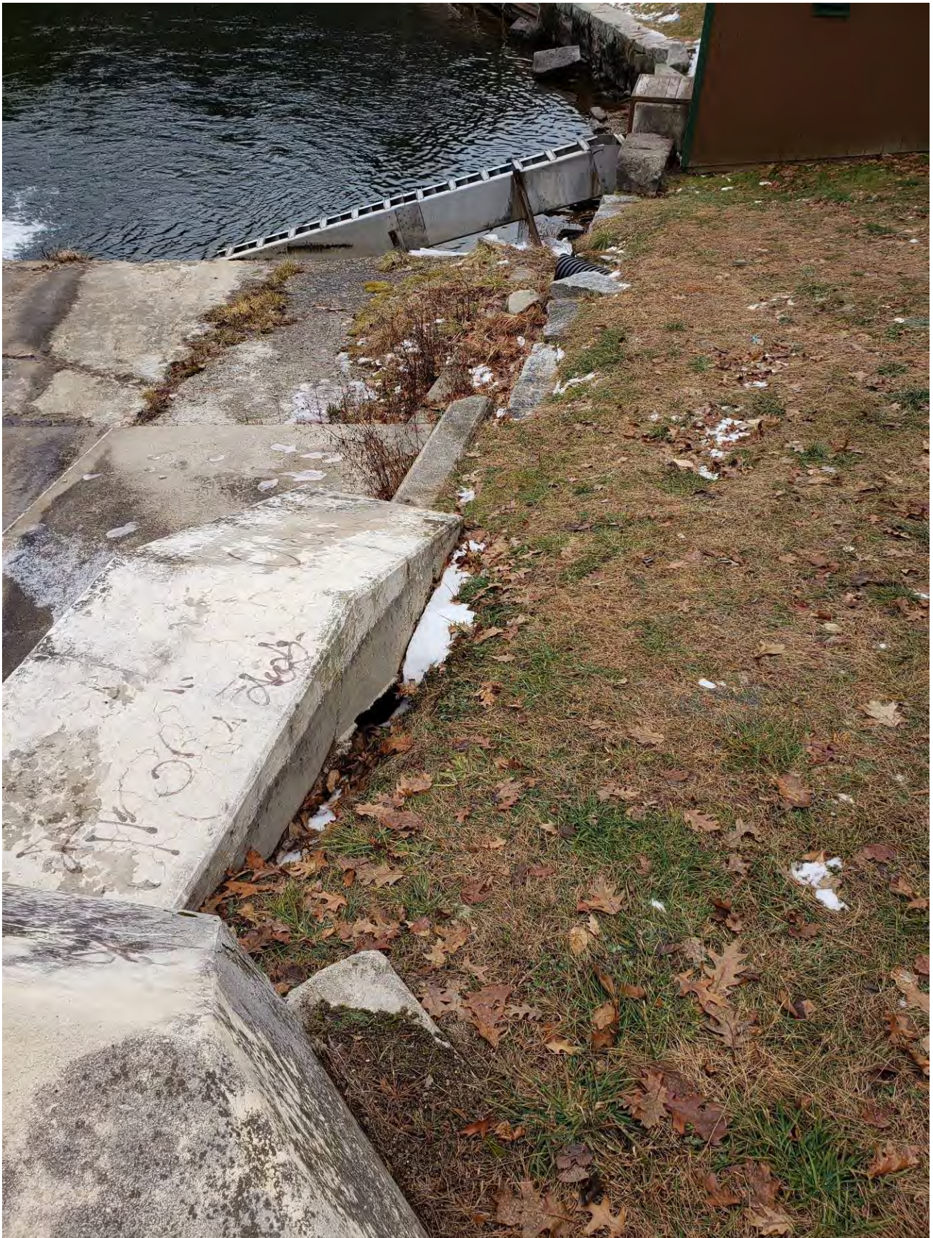
PHOTO 27: SEEPAGE AND LOSS OF SOIL ALONG RIGHT ABUTMENT DOWNSTREAM RETAINING WALL (1).
