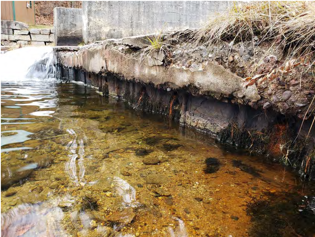
PHOTO 34: STEEL PILING BELOW END OF SPILLWAY APRON.
