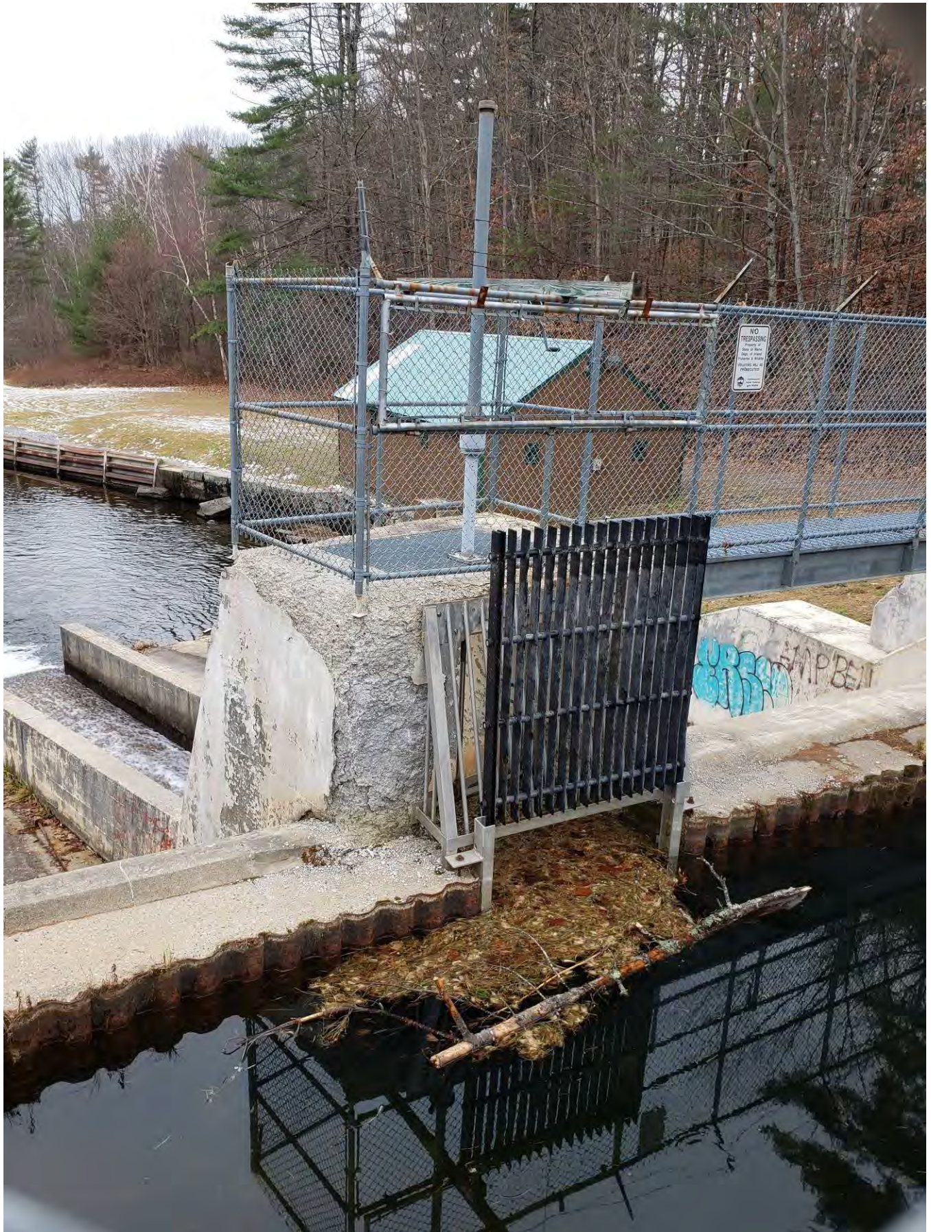
PHOTO 18: CONCRETE DEGRADATION TO LEFT SLUICWAY WALL.
