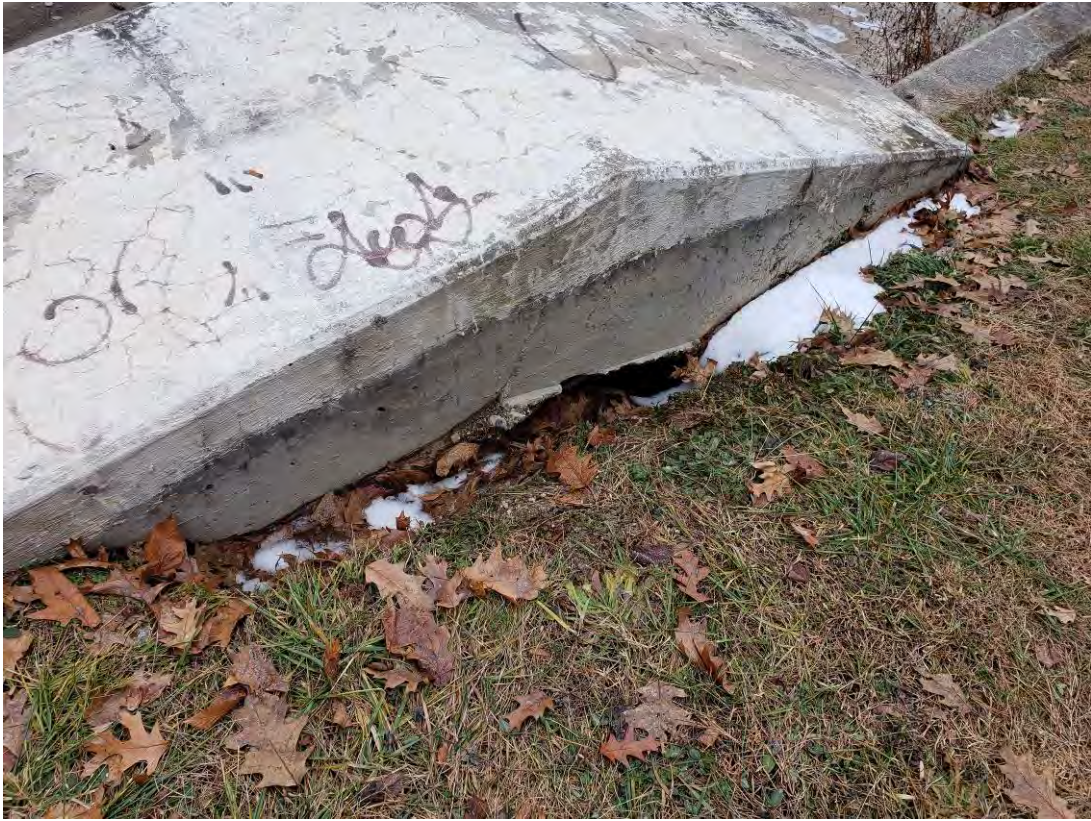
PHOTO 28: SEEPAGE AND LOSS OF SOIL ALONG RIGHT ABUTMENT DOWNSTREAM RETAINING WALL (2).
