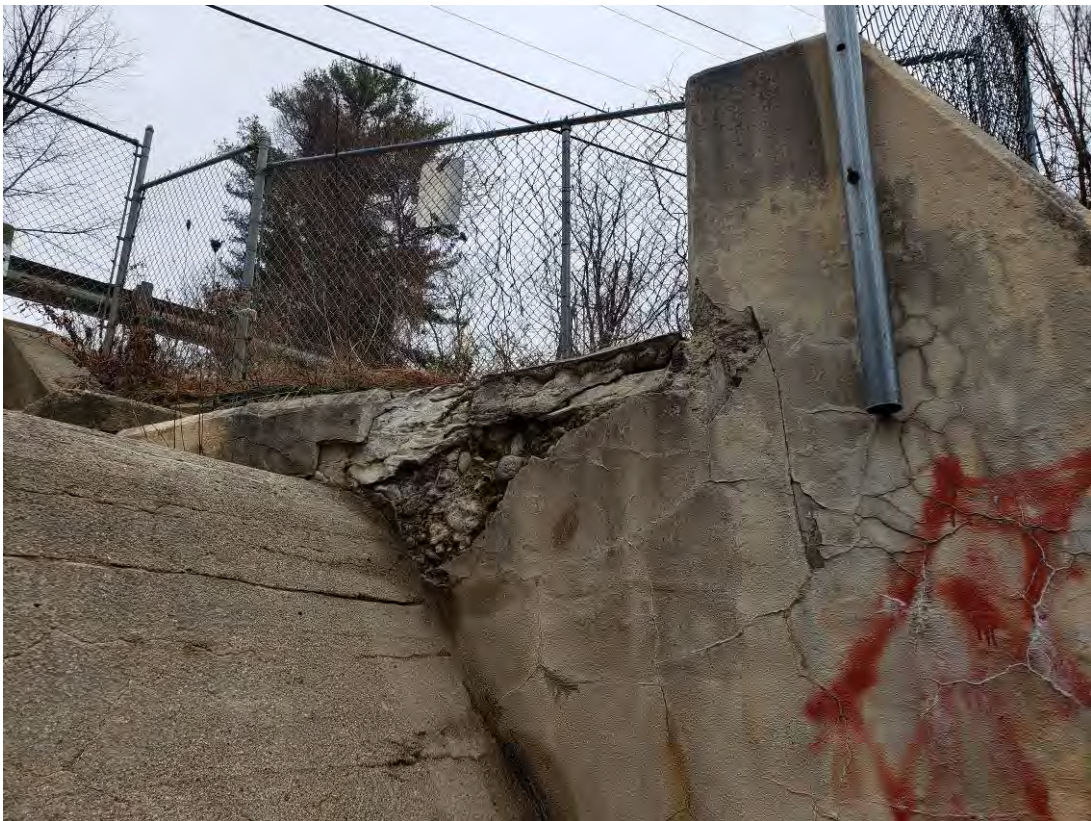
PHOTO 10: CONCRETE DEGRADATION TO LEFT ABUTMENT RETAINING WALL.
