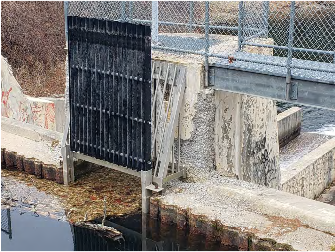
PHOTO 19: CONCRETE DEGRADATION TO RIGHT SLUCEWAY WALL.
