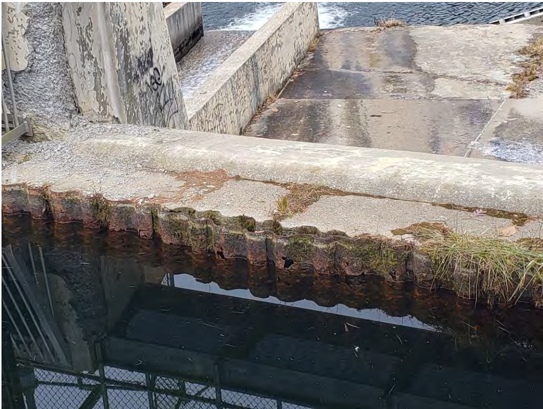
PHOTO 16: STEEL PILING CORROSION AND SEPARATION.
