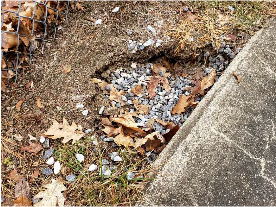
PHOTO 26: SINKHOLE UPSTREAM OF RIGHT ABUTMENT CUTOFF WALL.
