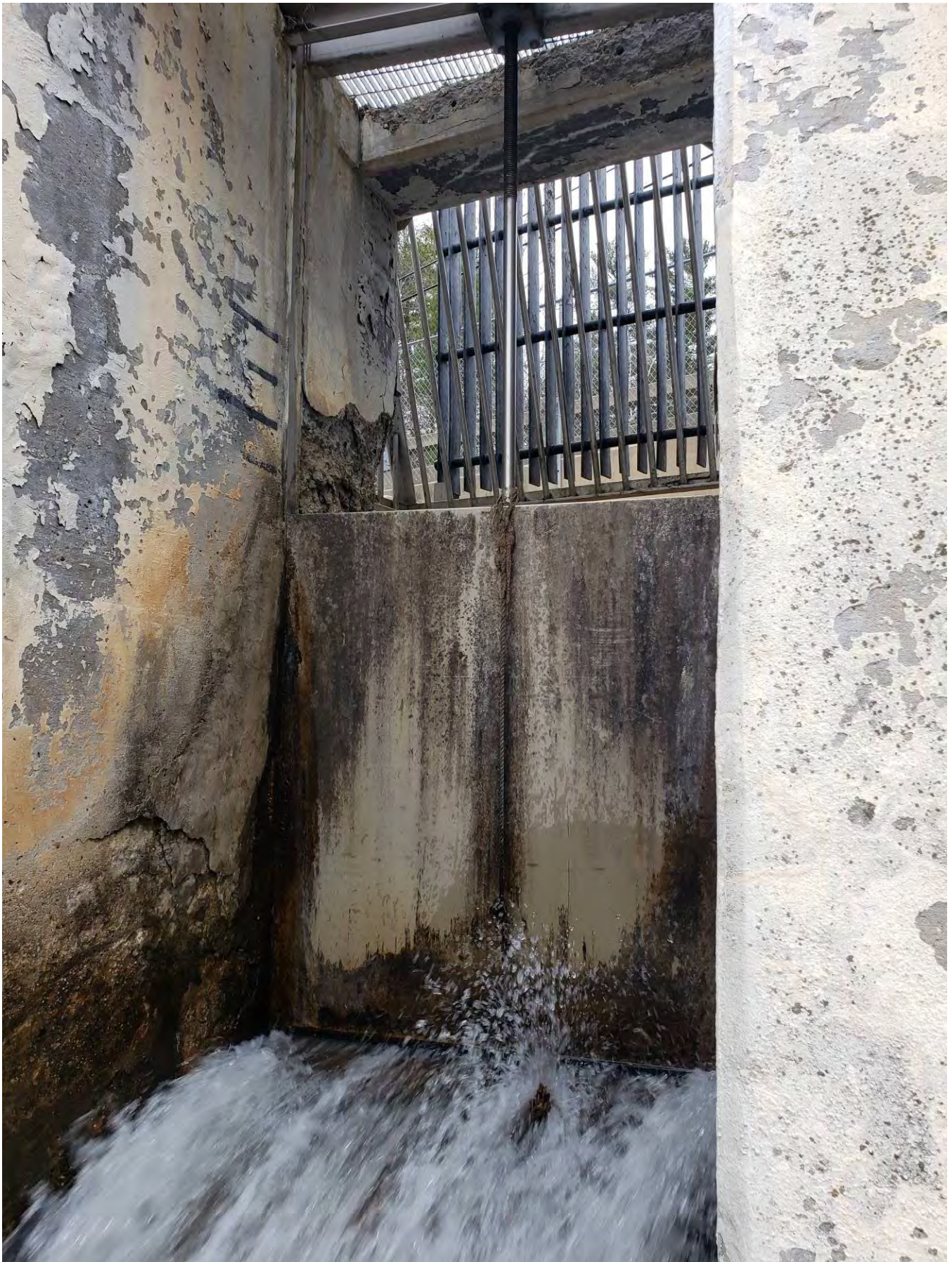
PHOTO 21: EXPOSED REINFORCING STEEL IN RIGHT SLUICWAY WALL.
