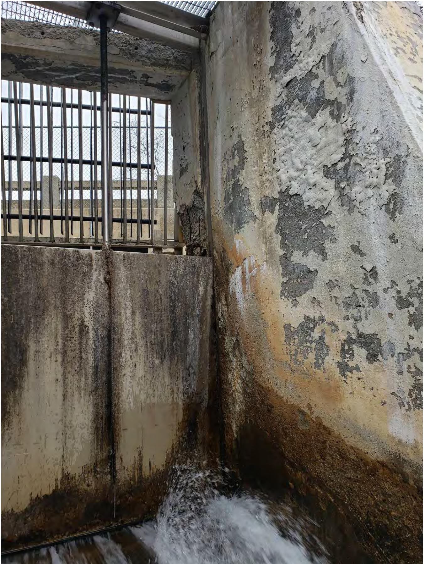
PHOTO 20: EXPOSED REINFORCING STEEL IN LEFT SLUICEWAY WALL.
