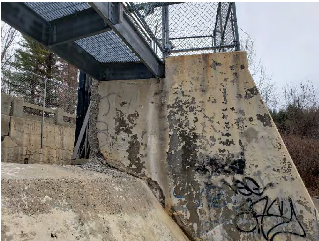
PHOTO 14: CONCRETE DEGRADATION ALONG RIGHT SPILLWAY AND SLUICEWAY INTERFACE.
