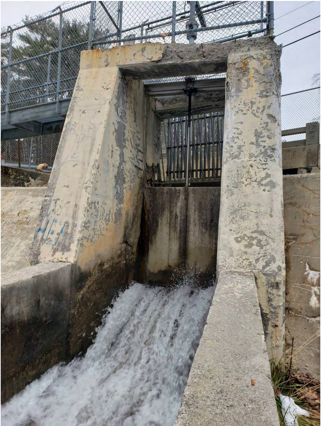
PHOTO 17: SLUICEWAY VERTICAL LIFT GATE AND CONCRETE DEGRADATION.
