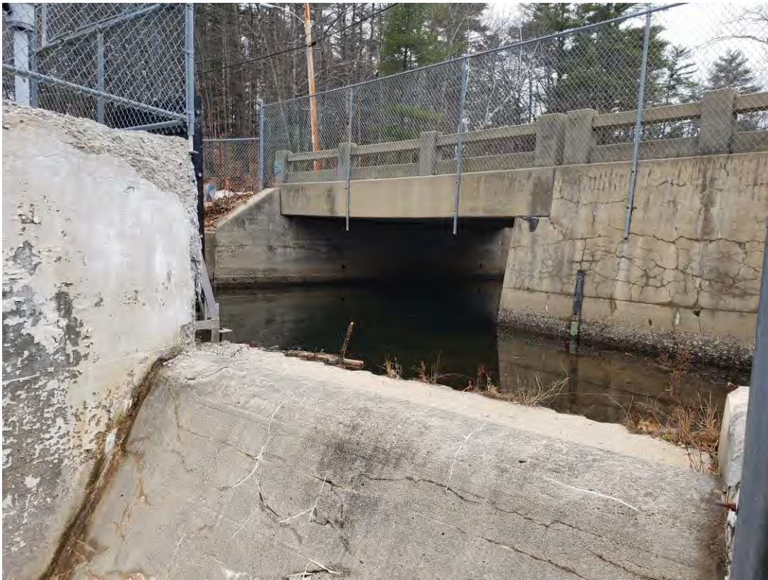
PHOTO 13: CONCRETE DEGRADATION ALONG LEFT SPILLWAY AND SLUICEWAY INTERFACE.
