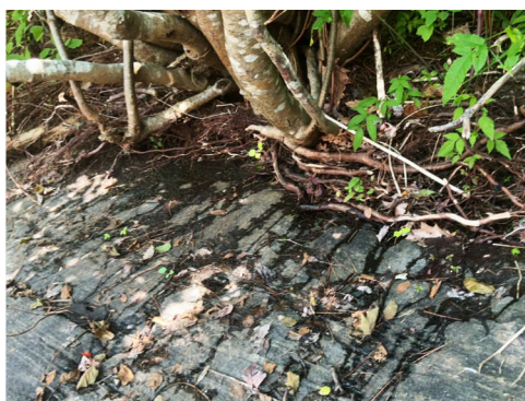
Evidence of a groundwater seep.
